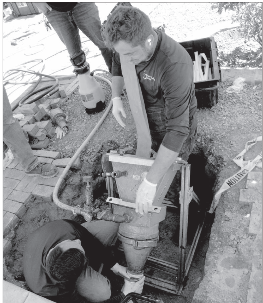
PIPELINERS – Plumbers Ruben Rodriguez, in the hole, and company owner Adrian De La Rosa insert a pipe lining material that helps create a pipe within the existing pipe. This pipelining is created out of a special epoxy and maintains the strength of a new pipe.
